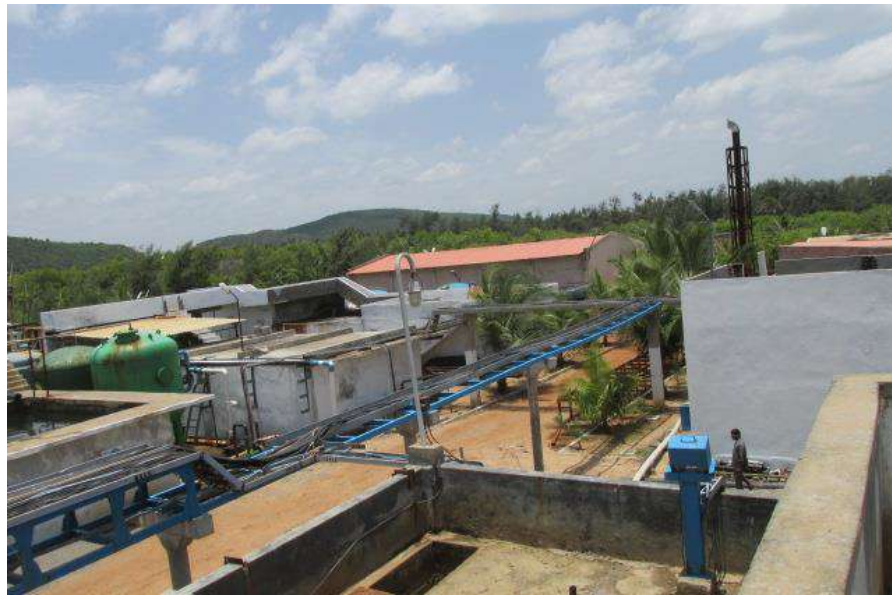
Fig. 1.3: Desalination plant in the Hetero Premises
