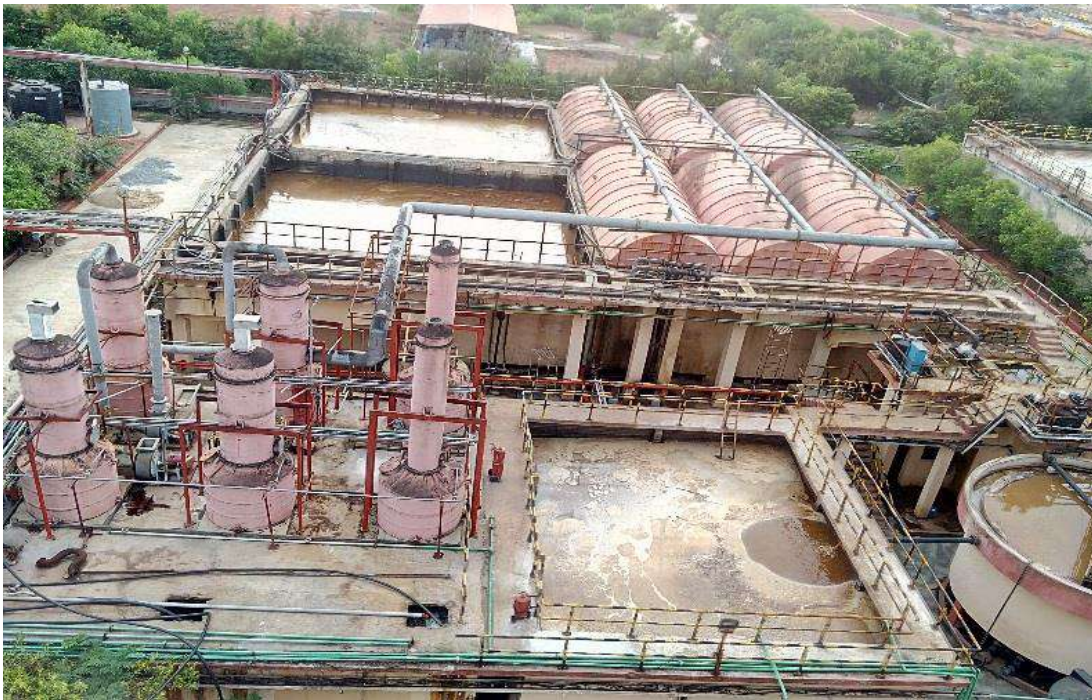
Fig. 1.8: HTDS Tanks covered with Hoods and connected to Scrubbers
