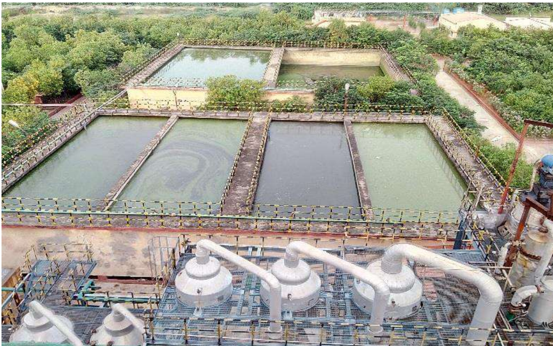
Fig. 1.10: Guard ponds for storage of treated Effluent
